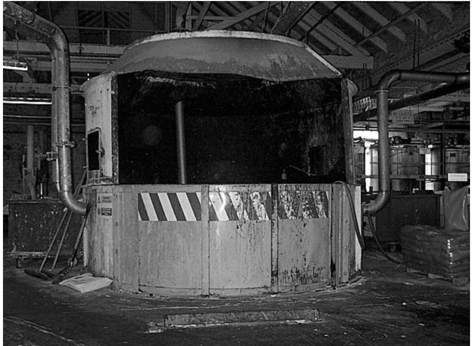
Figure 13 The fencing around open-topped pulpers should be designed so that people cannot climb onto it
