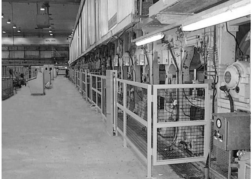
Figure 23 In some mills, interlocked distance guarding is being developed
