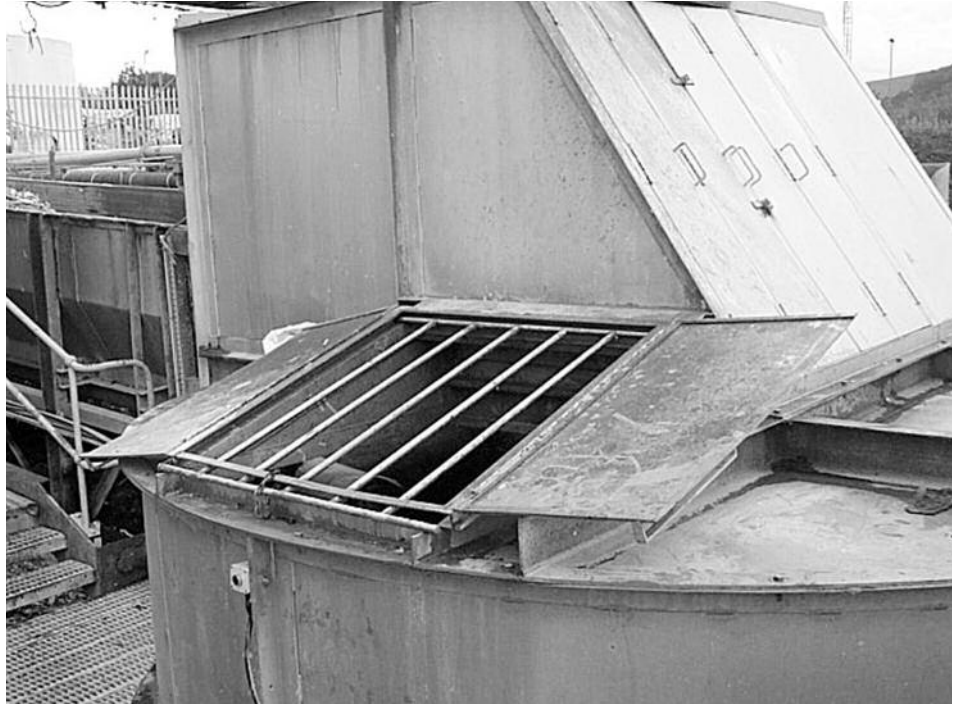
Figure 12 Pulper with fixed grille on hatch to prevent people falling through
